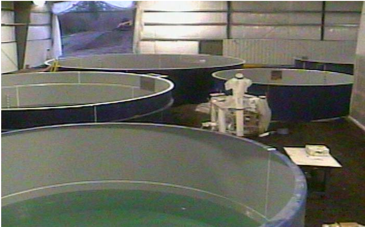
New 400k lbs. Recirculation Facility at Rochester
